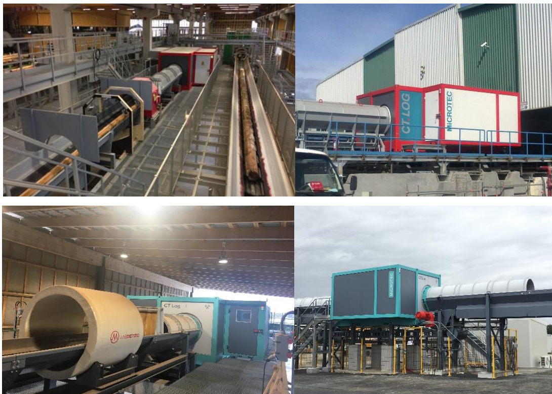
Figure 3.35 Some CT Log installation: from top left Siat-Braun (France) Arauco (Chile) Fiskarheden (Sweden) Piveteaubois (France).
