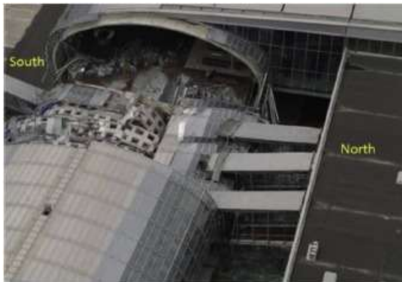
Figure 4. Collapsed zone of Terminal 2E at Charles de Gaulle Airport in Paris (5)
