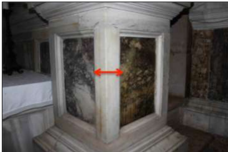
Figure 9.12: Dark coating seen on the marble panel on the right probably a past protective treatment.
